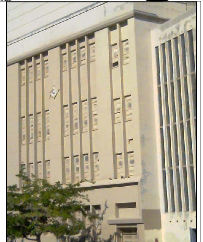
Reno Lodge is getting an exterior face lift. The building is being painted tan.
